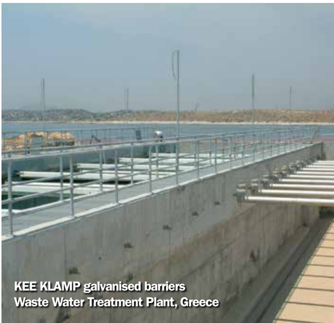
KEE KLAMP galvanised barriers Waste Water Treatment Plant, Greece
